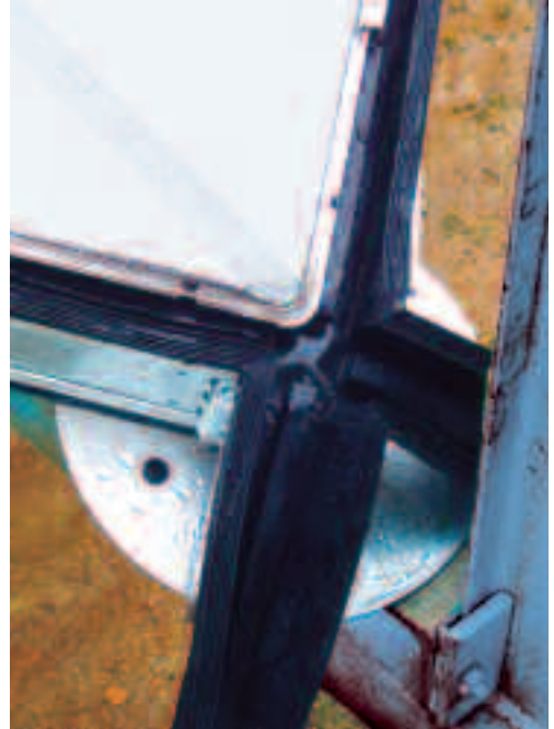
Figure 18: The stainless steel outer panel is insulated from the inner galvanized steel panel by suitable joints.
