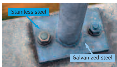
Figure 8a, 8b: Stainless steel fasteners on much larger galvanized steel components do not normally cause corrosion.
