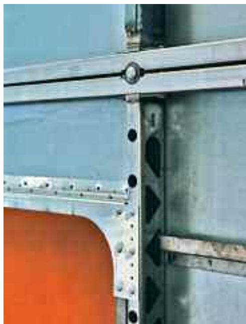
Figure 24: In this side wall of a commuter train, the structure and outer panels are in different grades of stainless steel. As these have identical potentials, no galvanic corrosion can occur.
