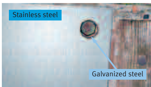
Figure 10a, 10b: Practical examples of the principle shown in Figure 9 (galvanized carbon steel in contact with stainless steel, in a marine atmosphere)
