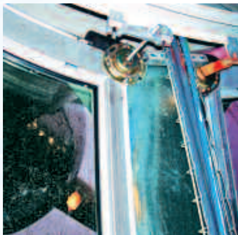
Figure 20: To prevent galvanic corrosion, the stainless steel cladding is fastened to the carbon steel inner structure in non-humid areas.
