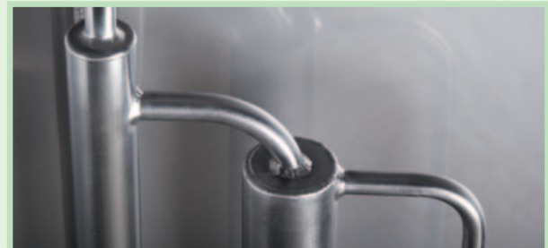
The fully air-tight design involves stainless steel valves and piping, which must resist atmospheric pressure
