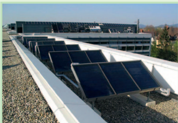
Solar hot water panels just 20 m 2 in size are sufficient to provide energy for the cooling process
