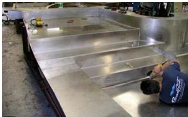
The ease of welding and polishing is a benefit when pools have to be assembled on site.
