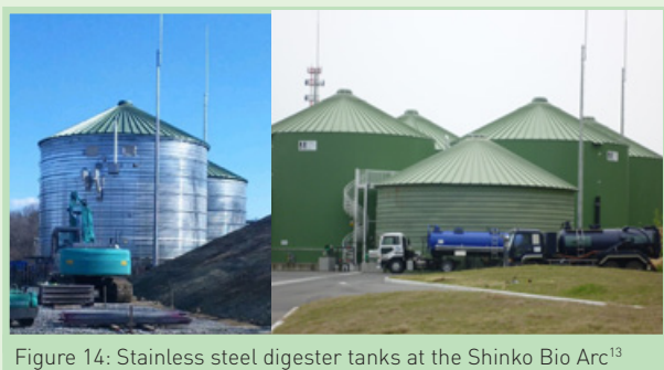
Figure 14: Stainless steel digester tanks at the Shinko Bio Arc 13
