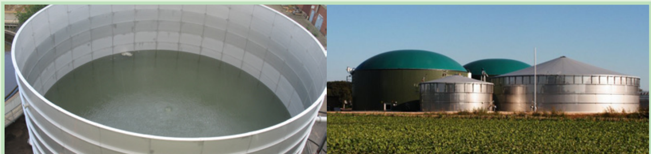
Figure 7: Interior view of stainless steel storage tank (left) and exterior view of storage and digester tanks 6
