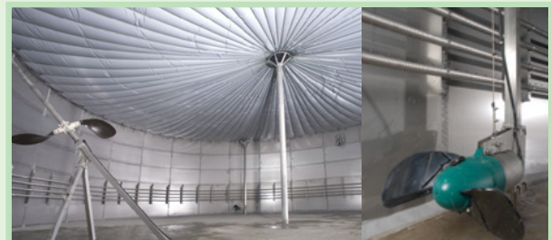
Figure 8: Inside view of a stainless steel digester tank 7
