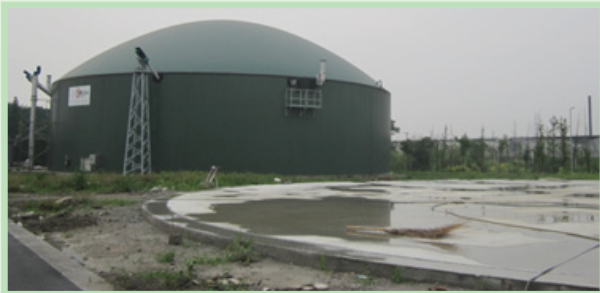
Figure 11: Digester tank in the Wuxi Kaipu CNG System 10
