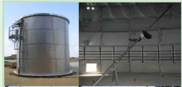
Figure 12: Frankfurt Hahn Airport's co-generation plant showing a pre storage tank (top left), external view of the plant (bottom) and inside of a tank (top right) 11
