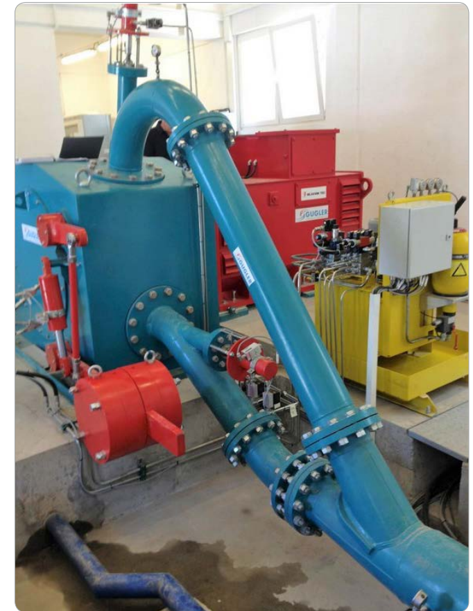
Micro Pelton Turbine, Gradecka, Macedonia Power: 936kW Head: 304 m Flow:0.35 m 3 /s Picture courtesy of Gugler GmbH, Austria
