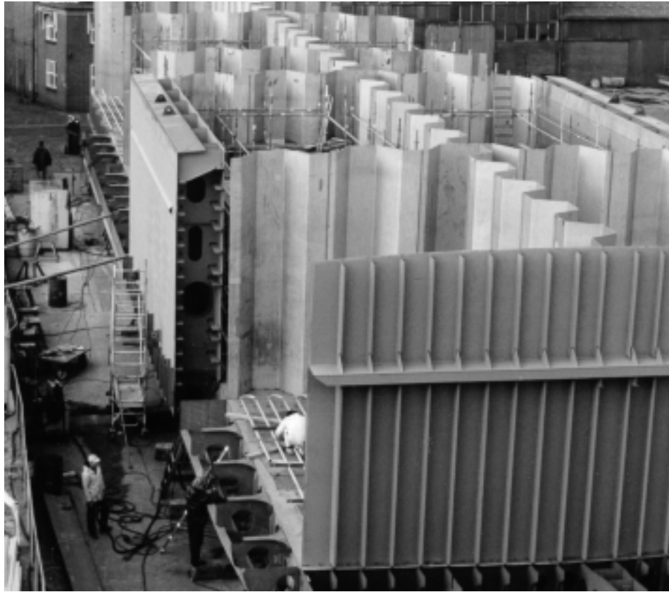
Figure 2. Actual view of the layout of the tanks.
