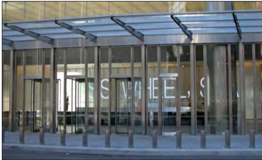
Blast resistant columns in entrance canopy, Seven World Trade Centre, New York
