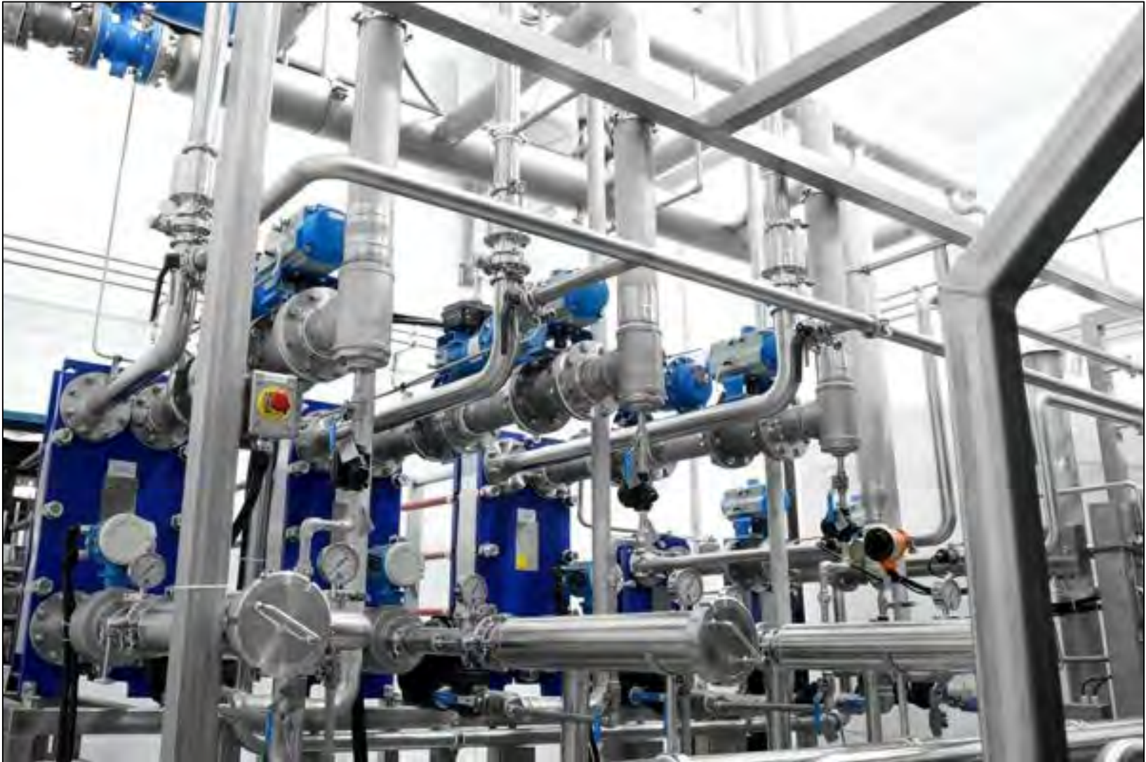
Stainless piping system
