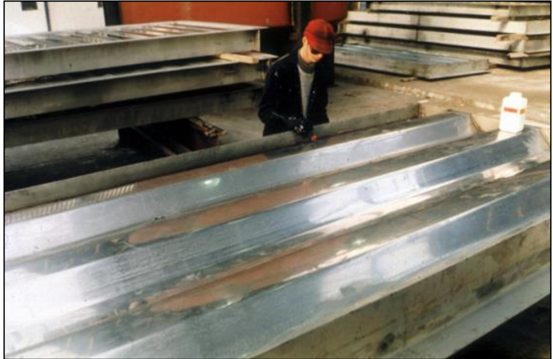
A trapezoidal blast resistant wall being fabricated for the topsides of an offshore platform
