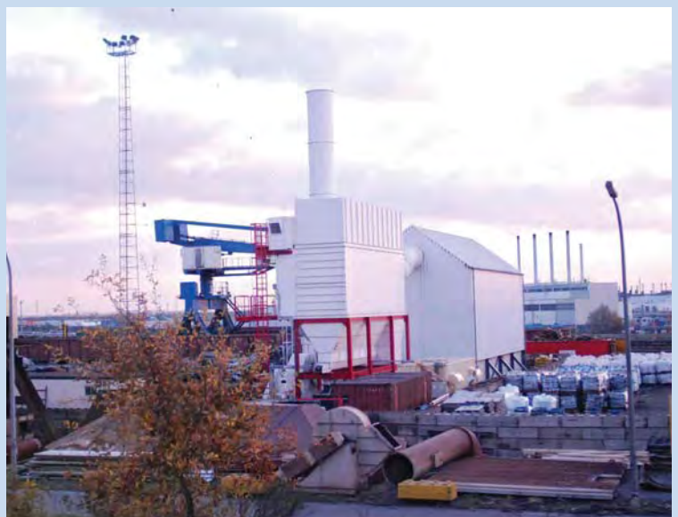
Aperam Genk de-dusting plant
