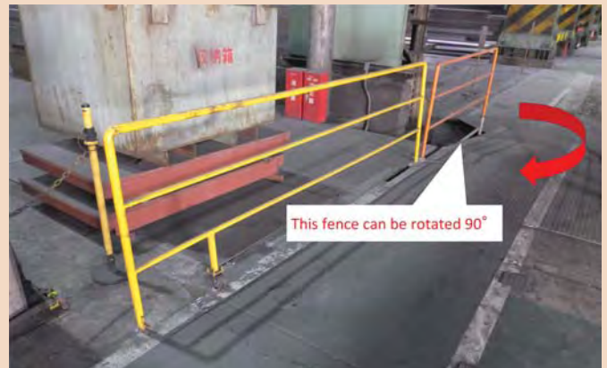
4. A movable barrier prevents pedestrian access during vehicle movements
