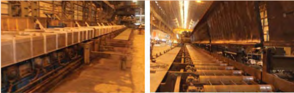
Retractable heat retention cover at RM exit side (left shows down condition, right shows up condition)
