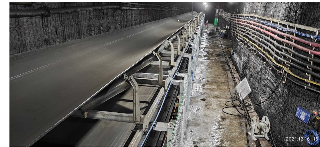
Figure 5: Stainless steel rollers and supports for coal belt conveyors (Newly developed stainless steel)
