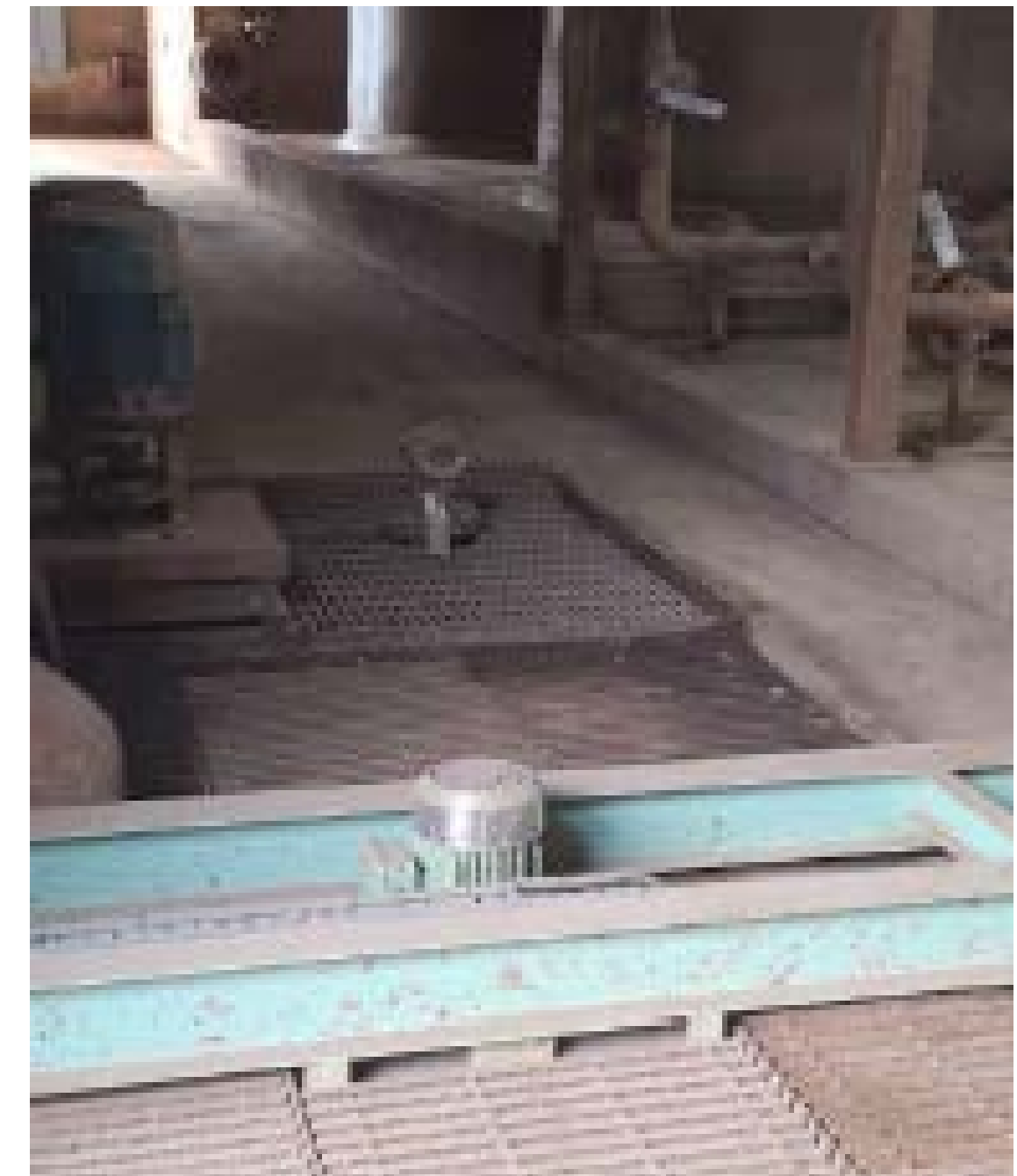
Picture of the Agitator at sump pit 7
