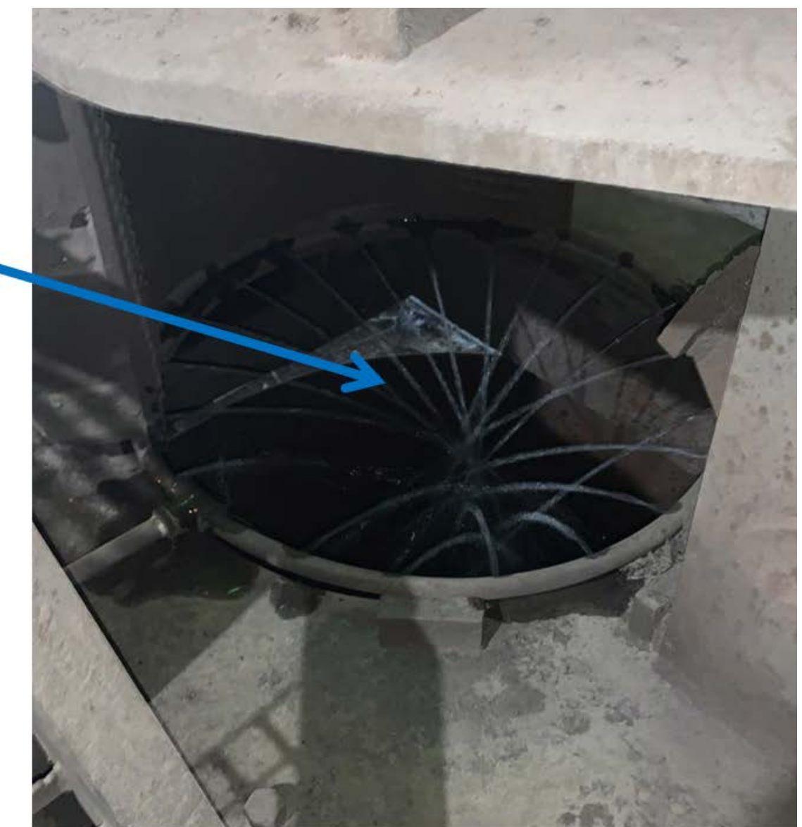
Cooling water that is sprayed onto the electrode
